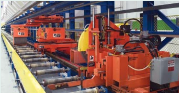
The Twin Puller with Adjustable Hot Saw is installed in a double-length configuration. Each puller head has its own 20 HP A.C. Vector drive, and pulling tension can be adjusted from 50 to 1000 pounds.
